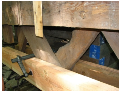
One of the lattice truss timbers showing damage from porcupine.
