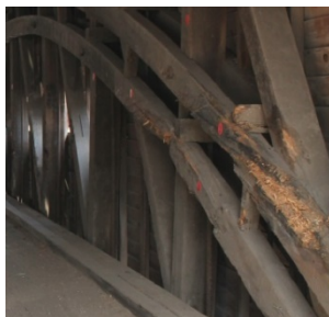
Photo of Truss Damage Courtesy of Lancaster County Timber Frames, Inc.
