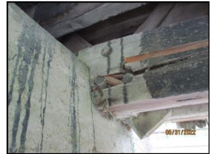
Connection of the lower chord at the abutment on the northwest corner.
