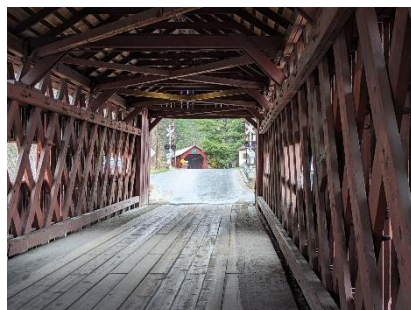
Interior of the Northfield Station Bridge with the Lower Cox Brook Bridge in the background
