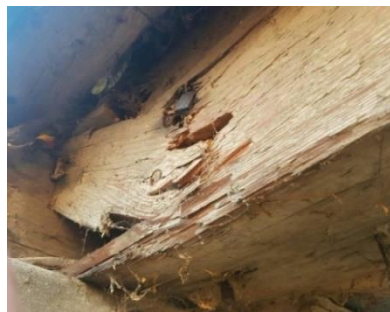
Broken lower chord at the west end of the bridge.
