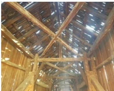
Holes in the roof before repairs.
