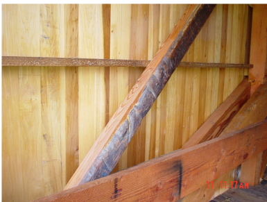
Interior of the Walcott Bridge showing the slice of historic wood glued onto a new timber beam.
