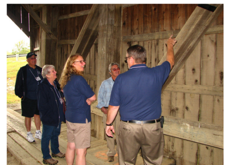
VP Karl Olson pointing out the high water mark in the Grange City Bridge
